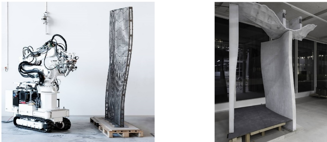
Fig. 3. Prototype of double-curved wall built with the Mesh Mould process. IF and MMW (left) and finished wall (right). (Source: [42].)
